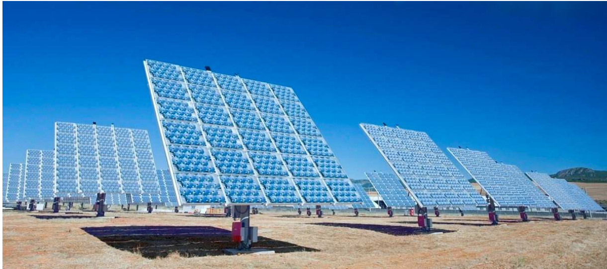
Figure 1. SolFocus SF1000 HCPV modules in installed array format.
